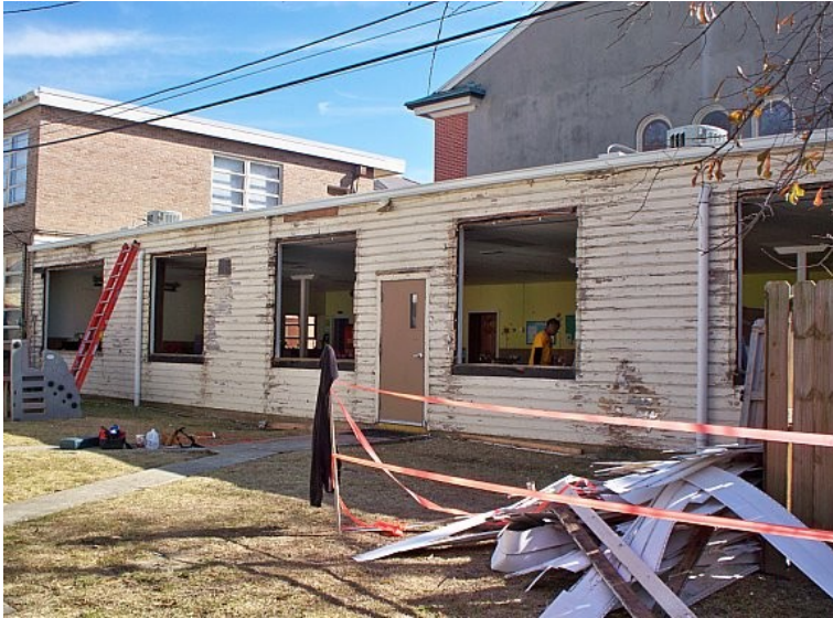
The side (Day Care side) of Fellowship Hall before windows and siding
